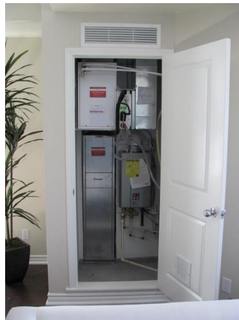
Installed Combo System
